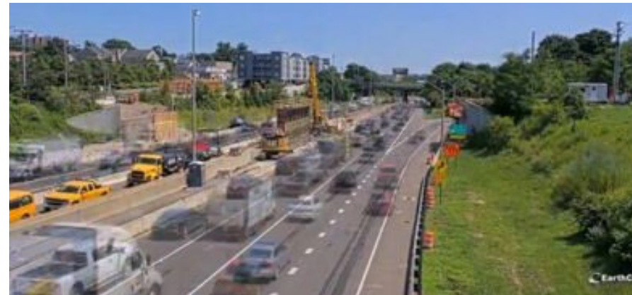
A timelapse photo of the Fairfield Avenue bridge over I-95 in Norwalk as it was being reconstructed after being demolished after a fiery accident in May. Photo courtesy of Gov. Lamont's office
