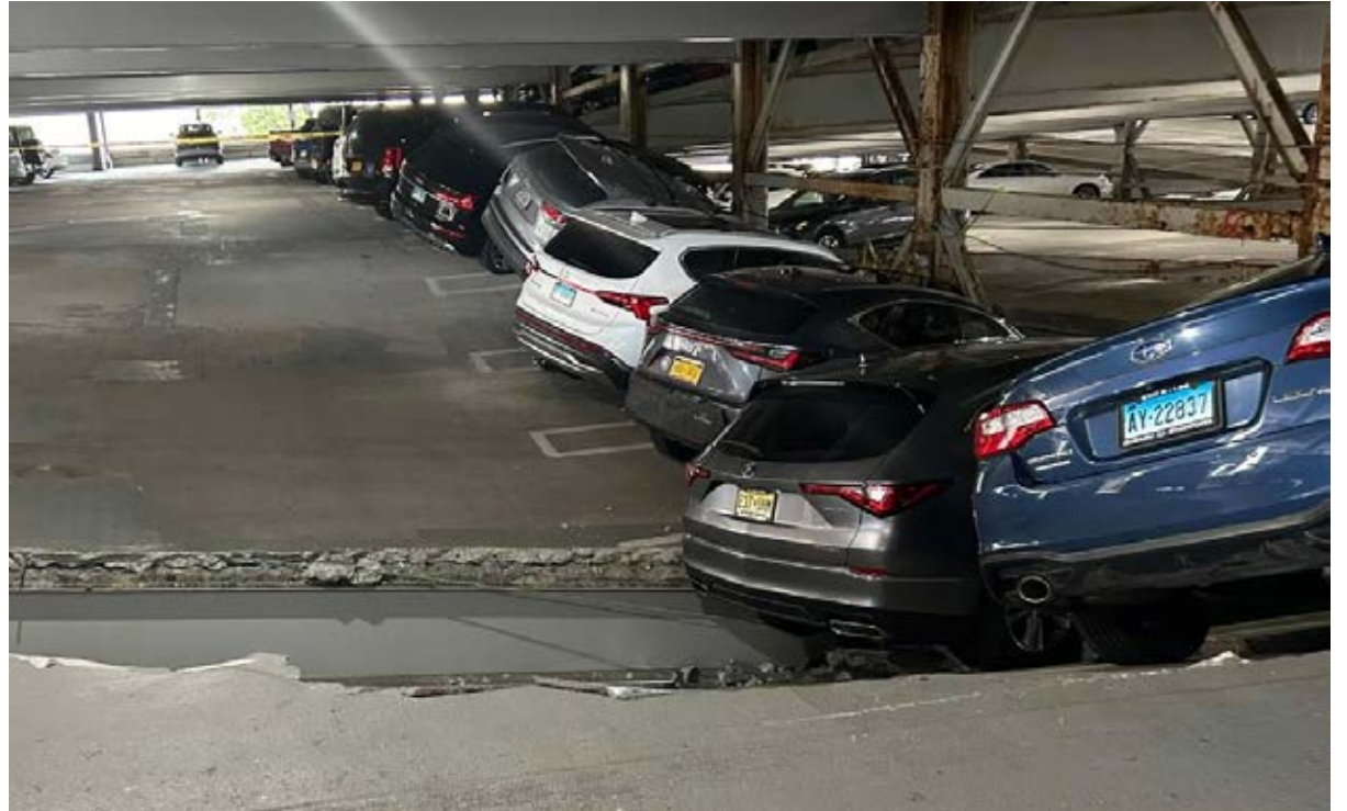
Damage inside Hale Avenue garage. Yonkers Fire Department photo.
