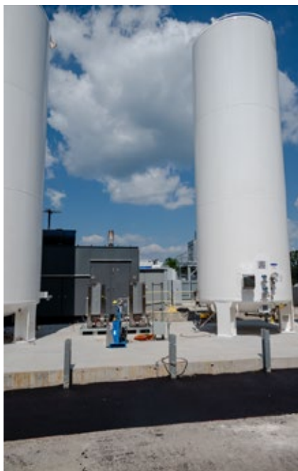
Tanks which will hold purified Carbon Dioxide captured from the demonstration plant being installed at Fuel Cell Energy's Torrington production facility.
