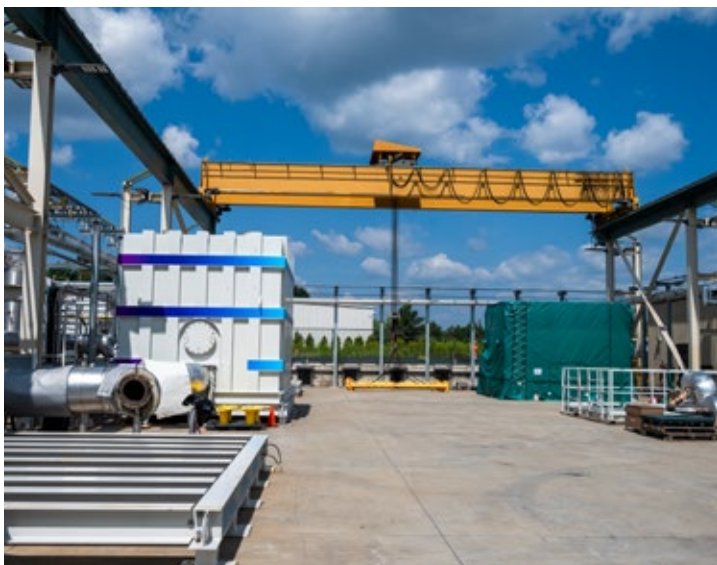
A fuel cell undergoing installation at a demonstration plant at Fuel Cell Energy’s Torrington production facility. Photos by Justin McGown.
