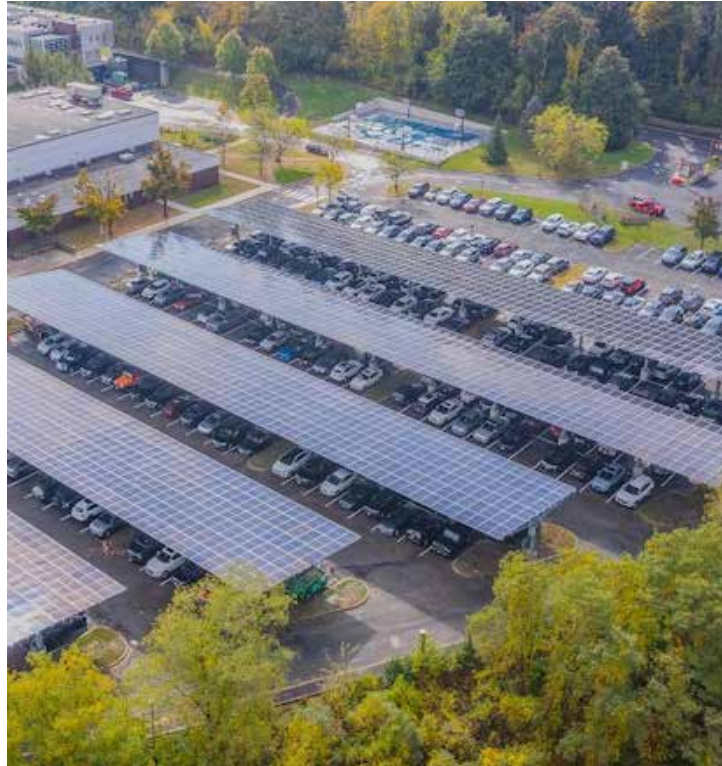
The new solar panel carport at Ridgefield High School will generate 1 MW of power annually. Photo courtesy of Ridgefield High School
