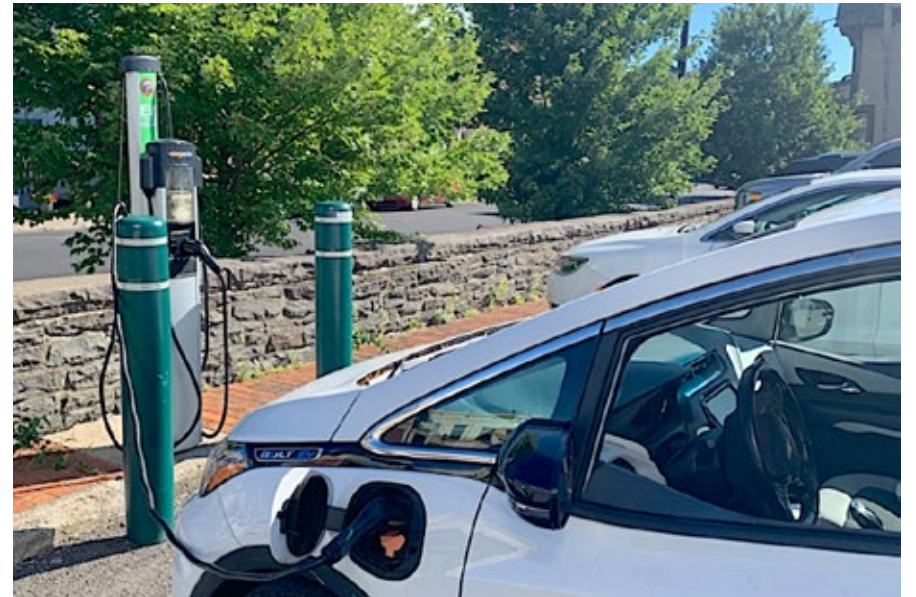
Solar charging station at Ulster County Office building.
