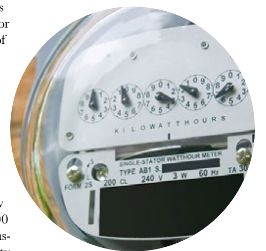
Electric meter, Central Hudson.
