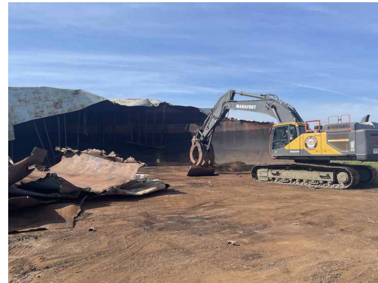
The demolition of one of the three large oil tanks at the decommissioned Manresa Island power plant. Photo courtesy of Manresa Island Corp.
