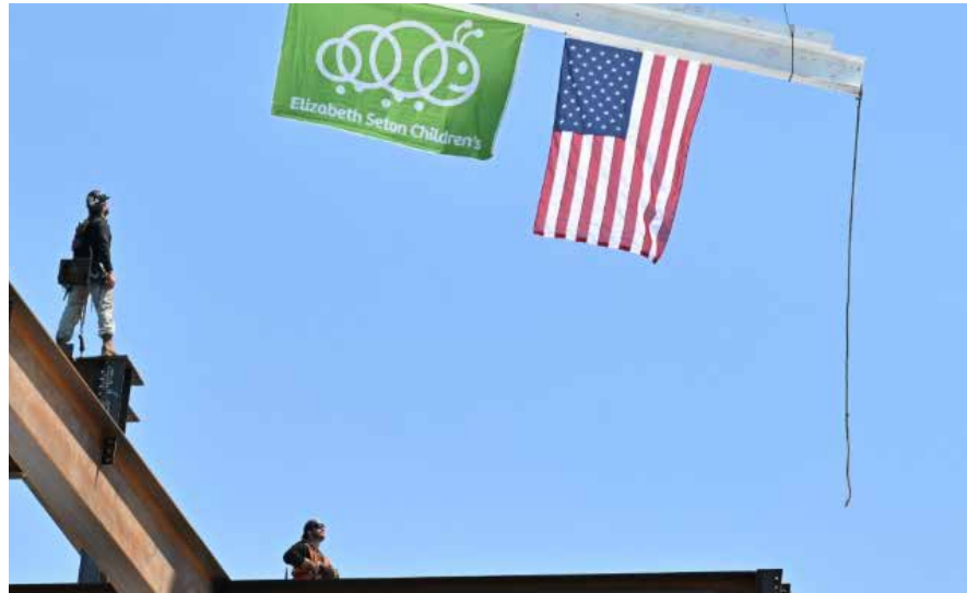
Final beam being put into position at Elizabeth Seton's new building in White Plains.
