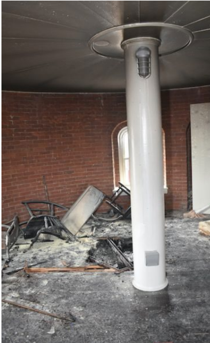
Some of the destruction at the Tarrytown Lighthouse. Photograph courtesy Westchester County Police.
