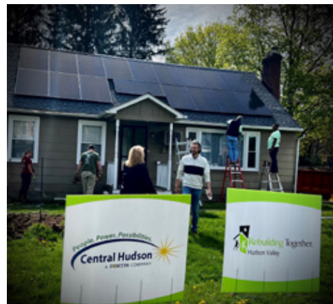
Volunteers make repairs to a senior's home during National Rebuilding Day in Poughkeepsie.
