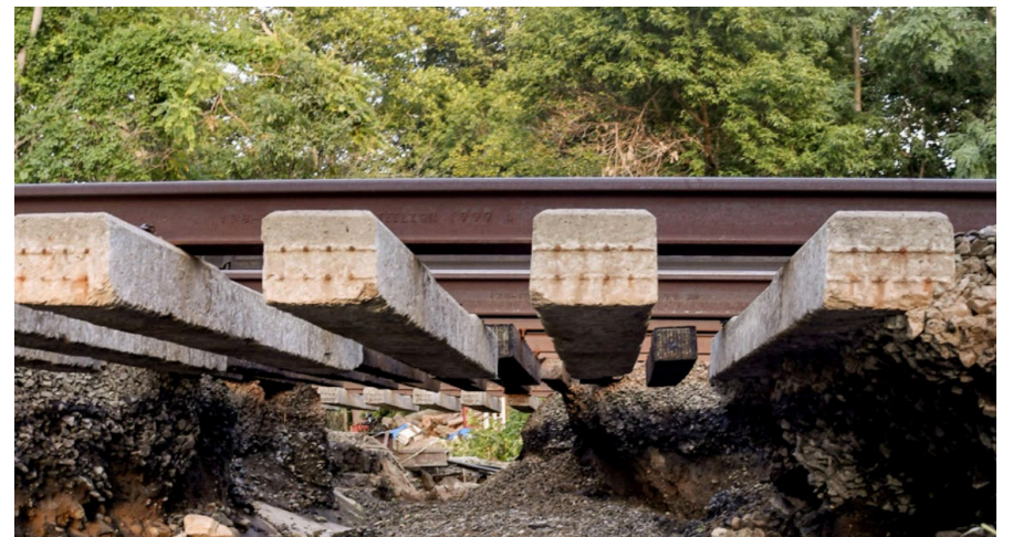
Dobbs Ferry track washout.
