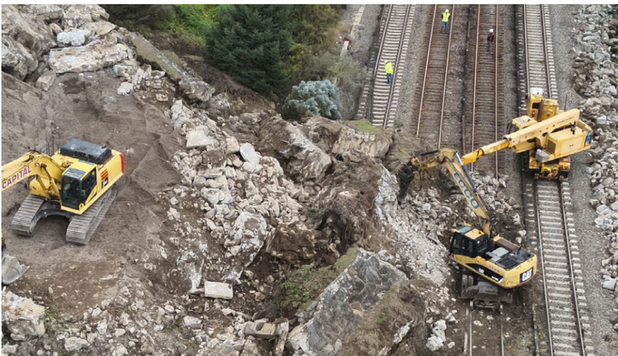
Aerial of track washout.
