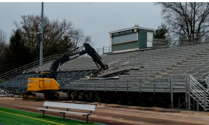
Demolition of the bleachers and Norman J. Sculley Press Box began immediately after the ground breaking.
