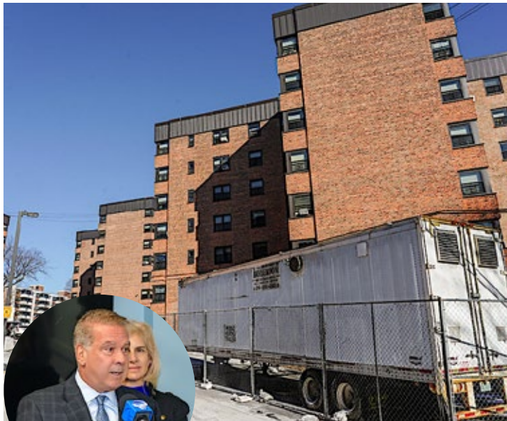
Palisade Towers complex. Portable boiler in trailer at right of photo.
