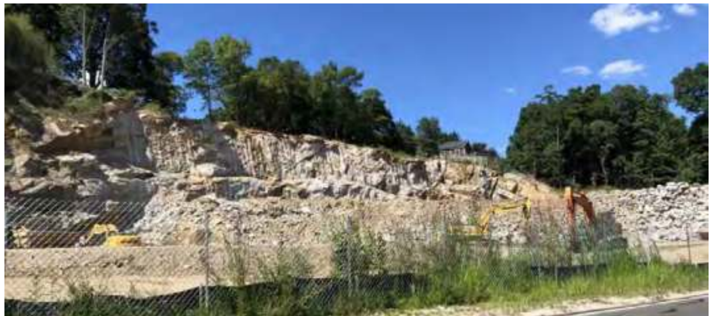
Work is underway to build a Brightview Senior Living facility at the site of a former quarry on Lake Street in Harrison. Photo by Peter Katz.
