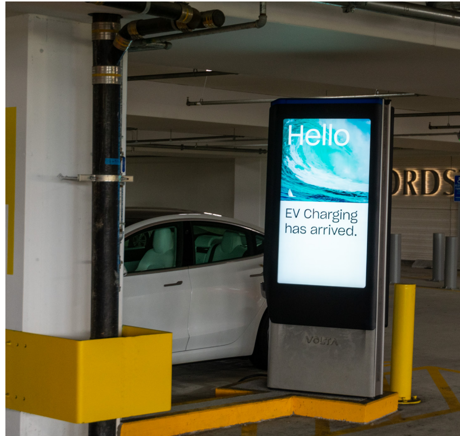
A Level 2 Charger installed at the SoNo Collection in Norwalk. Photo by Justin McGown.
