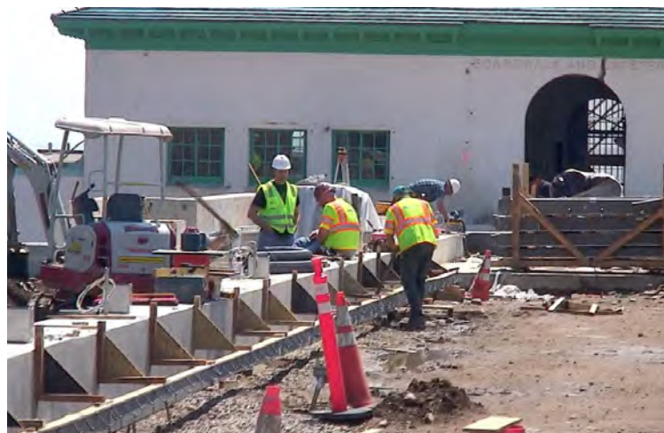
Construction workers at Playland on Memorial Day weekend. Photos by Peter Katz.
