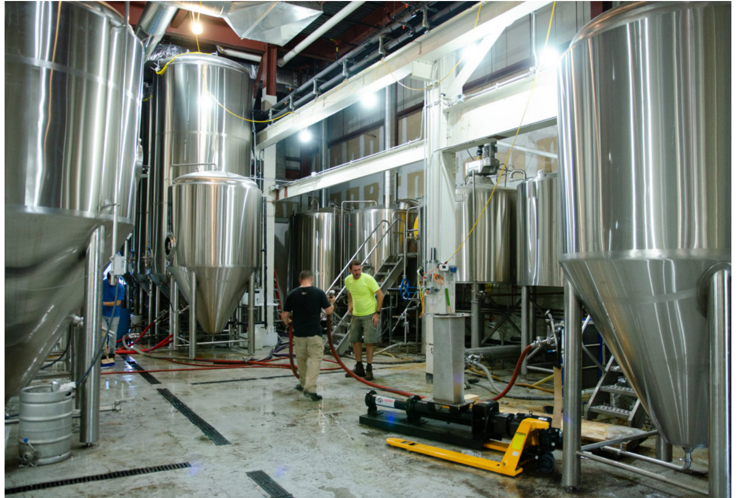
Sloop Brewing — some of the brewing equipment.
