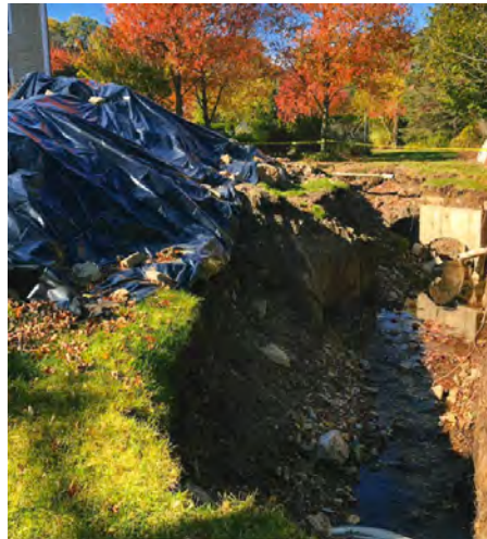
Pipeline in Harrison damaged by Tropical Storm Ida
